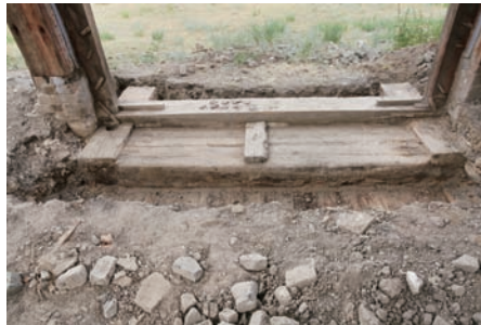
Side bottom of the eastern door
